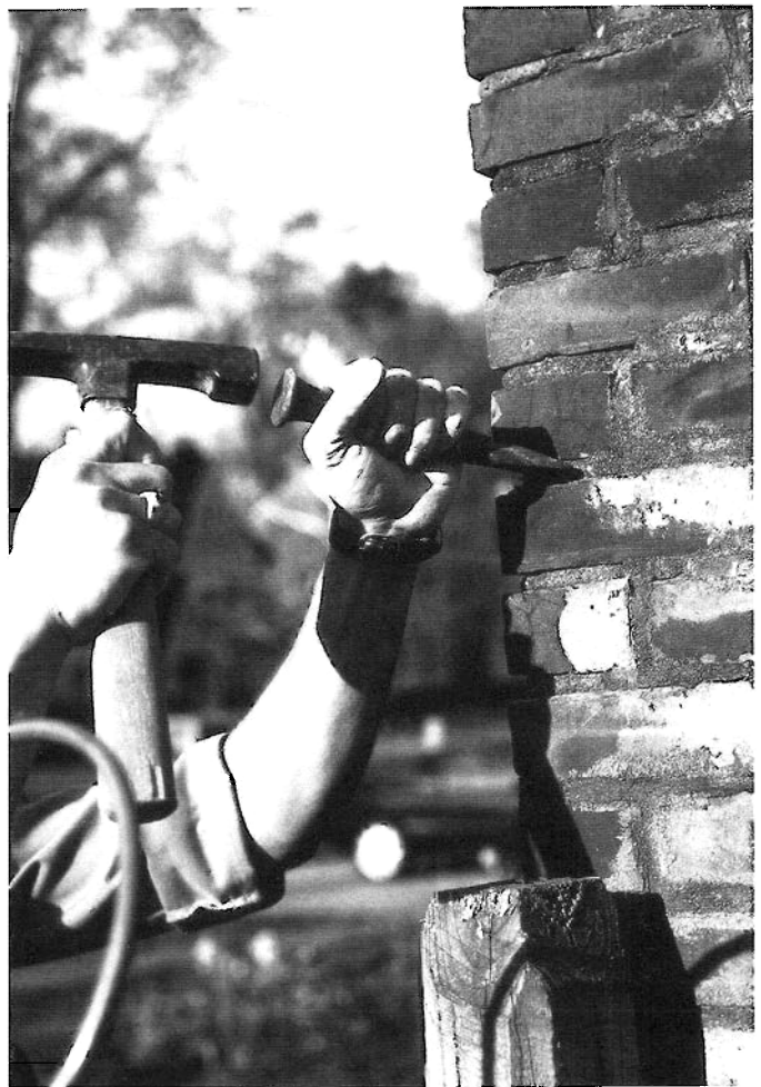
Figure 10. Using a hammer and masonry chisel is the least damaging and, thus, generally the preferred method of removing old mortar in preparation for repointing historic masonry. Photo: John P. Speweik.
