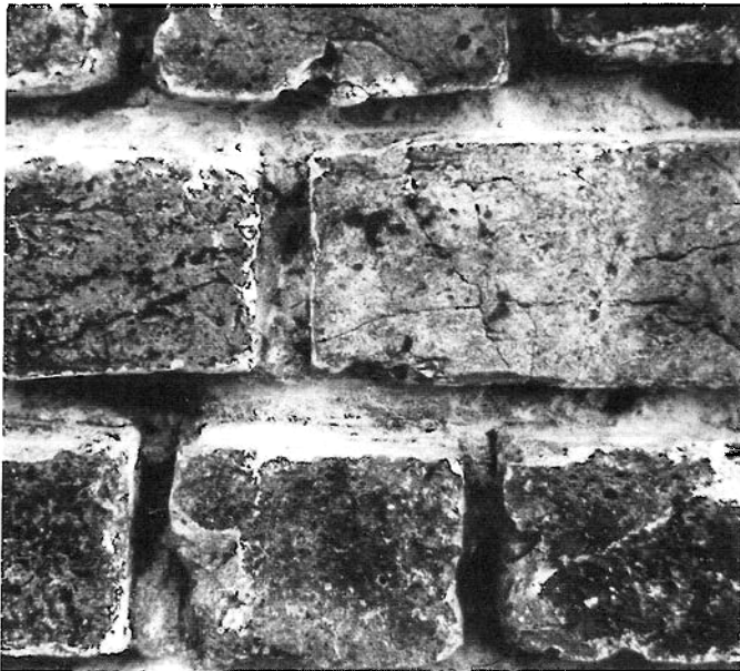
Figure 11. The damage to the edges and corners of these historic bricks was caused by using a mechanical grinder to rake out the joints. Note the overcutting of the head joint and the damage to the arises (corners) of the bricks. Photo: Lee H. Nelson, FAIA.
