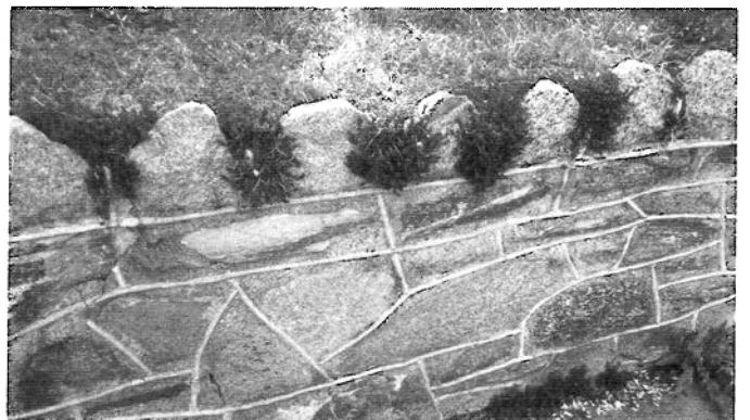
Figure 20. This stone garden wall was tuckpointed to match the tuckpointing on the c. 1920s house on the property. Photo: Anne Grimmer.
