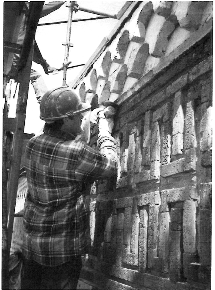
Figure 12 A power grinder, operated correctly by a skilled mason may be used in preparation for repointing to cut wide, horizontal mortar joints, typical of many early-20th century brick structures without causing damage to the brick. Note the use of protective safety equipment. Photo: Robert C. Mack, FAIA.
