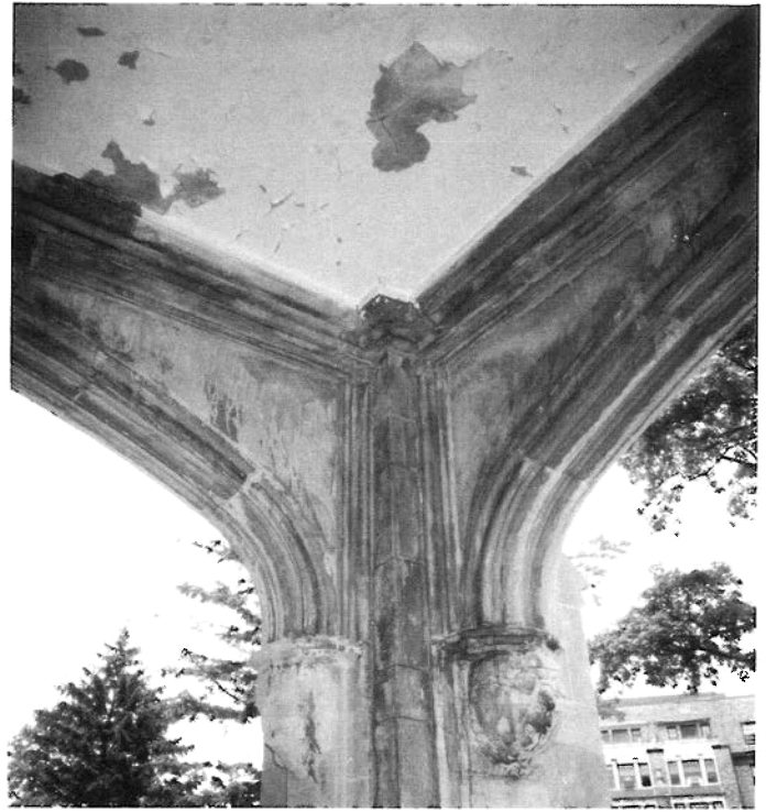
Figure 5. Repeated water washing did not remove the staining inside this limestone porte cochere. Upon closer examination, it was determined to be a water-repellent coating that had been applied many years earlier. An alkaline cleaner may be effective in removing it.
