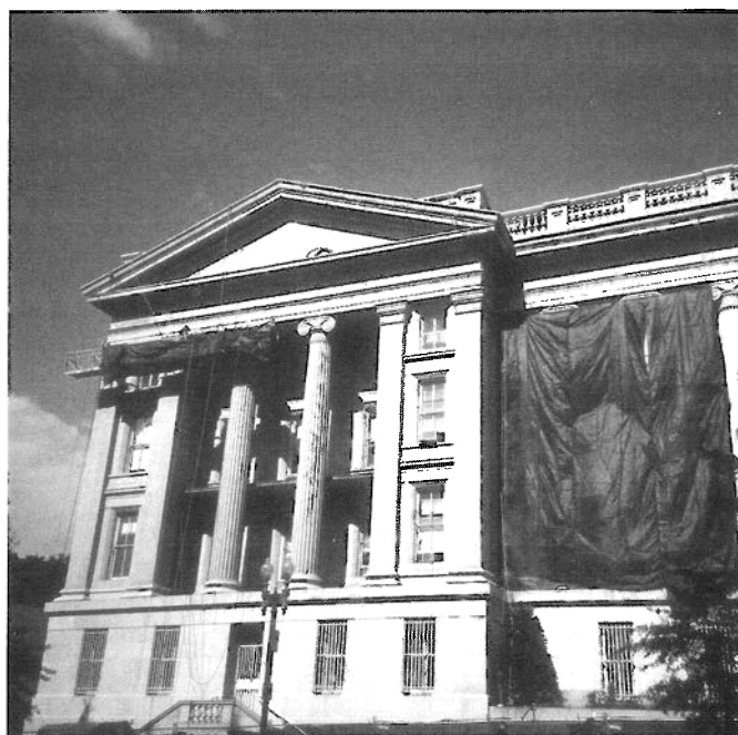
Figure 23. A tarpaulin protects and shields pedestrians from potentially harmful spray while chemical cleaning is underway on the granite exterior of the U.S. Treasury Building, Washington, D.C.
