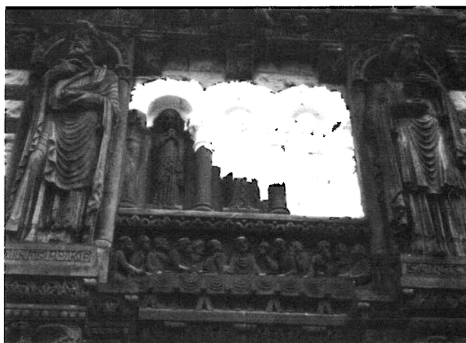
Figure 17. A poultice is being used to remove salts from the brownstone statuary on the facade of this late-19th century stone church. Photo: National Park Service Files.
