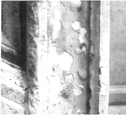
Figure 25. The clear coating applied to this limestone molding has failed and is taking off some of the stone surface as it peels. Photo. Frances Gale
