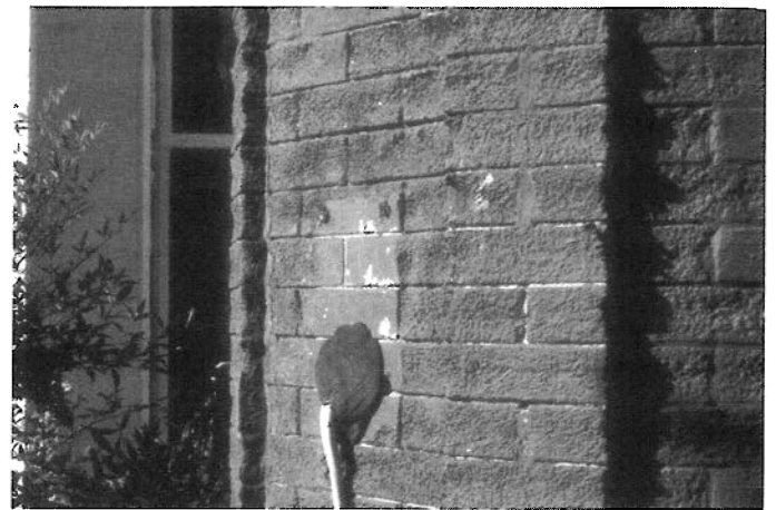
Figure 19. A comparison of undamaged bricks surrounding the electrical conduit with the rest of the brick facade emphasizes the severity of the erosion caused by sandblasting.
